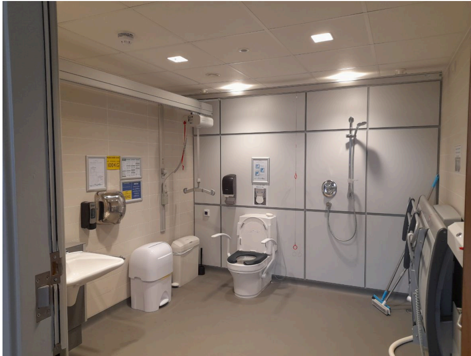
Changing Places toilet on Ground Floor.
